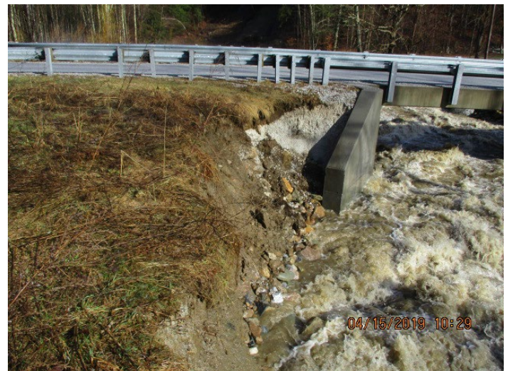
Fluvial Erosion Impacts to Bridge #25 over Mendon Brook on Medway Road – April 2019
